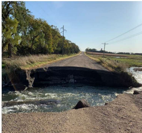
Figure 2. Work in water due to a road collapse may require US Army Corps of Engineers NWP or 401 or 404 depending on the method of repair. FEMA photo.
