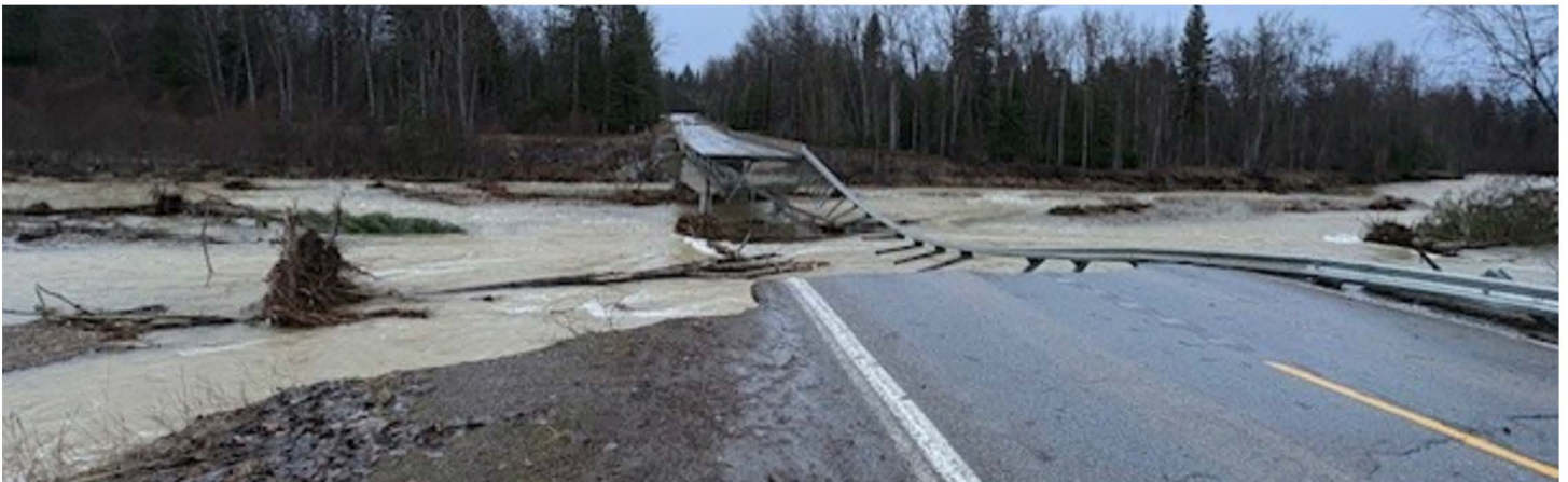
Above: Image of river flooding and bridge wash out in Lincoln County, MT following December winter storm and atmospheric river rain.
